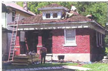
Work is already underway on refurbishing two homes in the Beacon Hill neighborhood. The homes on Tracy Avenue will be used as transitional housing for families forced to move out of their homes while they are refurbished.
